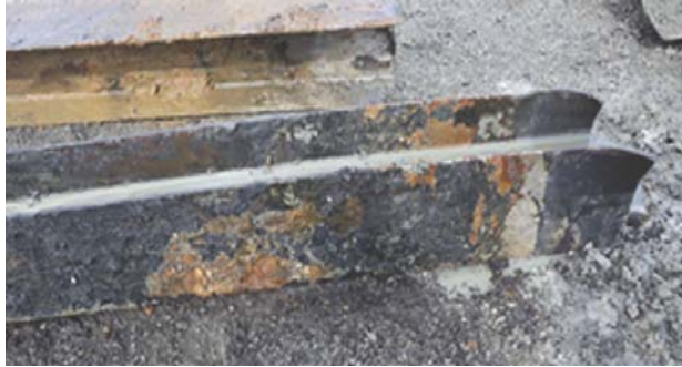
Figure 5 – Extracted abutment piles showing what appears to be a coal-tar epoxy coating and significant corrosion within the lower 300-600mm.
