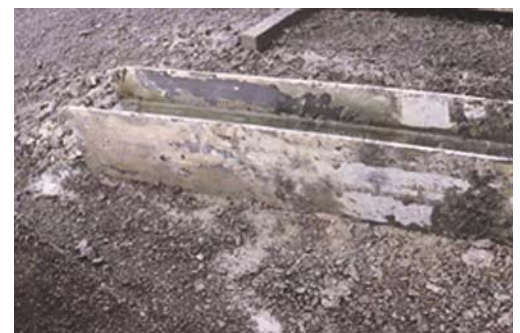
Figure 4 - Pile C2 showing no evidence of corrosion.
