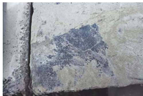
Figure 3 - Black bitumastic-type coating present.
