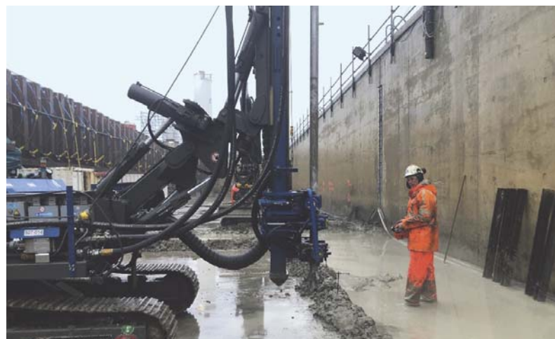
Figure 1 – Photo of the jet grouting rig on the relief platform in a temporary building pit.
