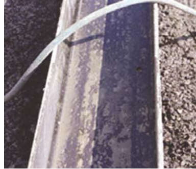
Figure 6 – The web of the A1 pile showing little sign of corrosion.
