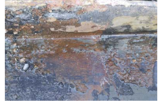
Figure 7 – The bottom 300mm of the A1 pile appears to be more heavily corroded with some scale being evident.
