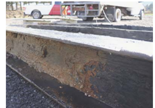
Figure 8 – Heavy corrosion scale near the bottom of the pile was noted on the web.
