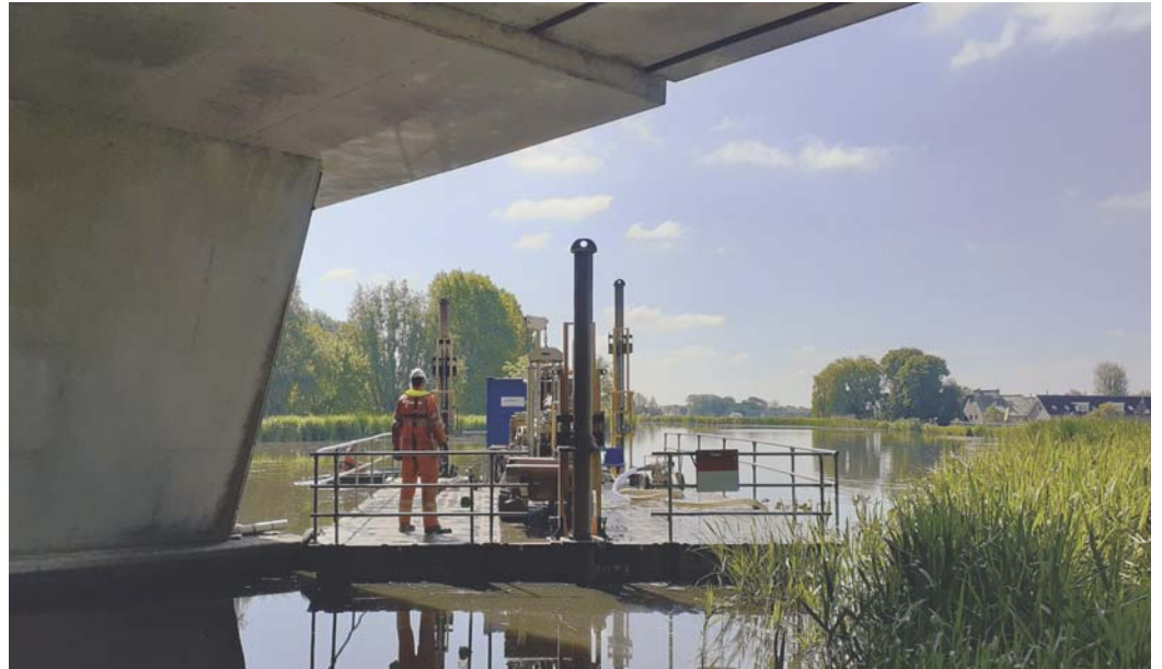
Photo 3 – CPTs also conducted on the water close to the existing pile foundations.
