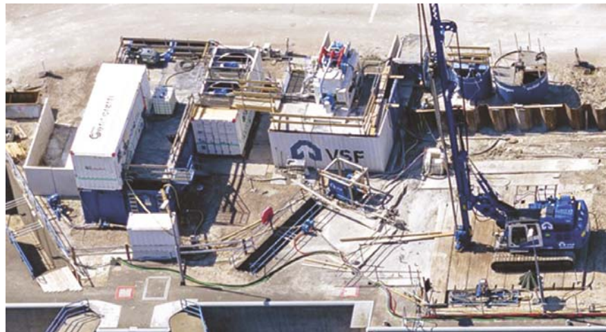
Figure 5 – Spoil treatment plant, with desander, centrifuge and small laboratory (Topview-fotografie).
